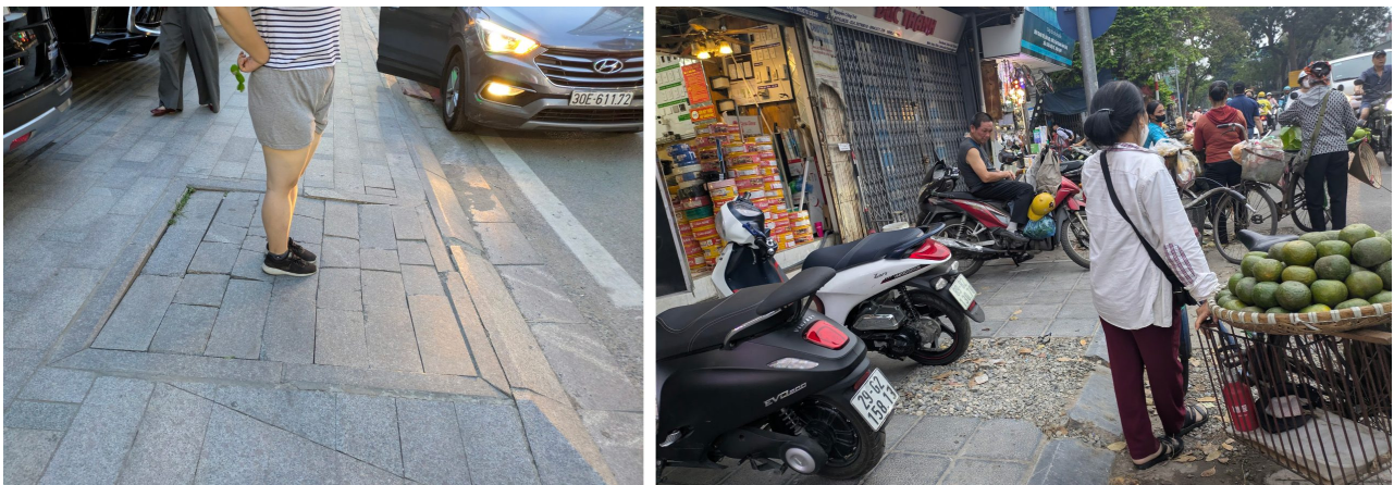
Left – Figure 7: A tree hole in front of the shopping mall was covered, May 2025. | Right – Figure 8: A tree hole in the local market, April 2025.
